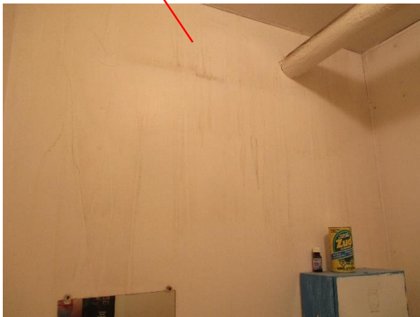
Water staining on bathroom wall. Approximate size of affected area 50 ft 2 .
