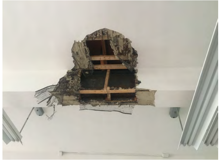
AREA ON THE CEILING TO BE REPAIRED
