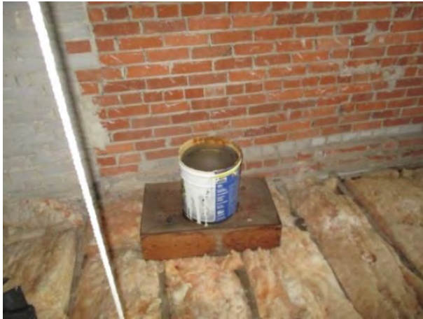
A bucket had been used to catch water drips from a hole in the roof below the bell.
