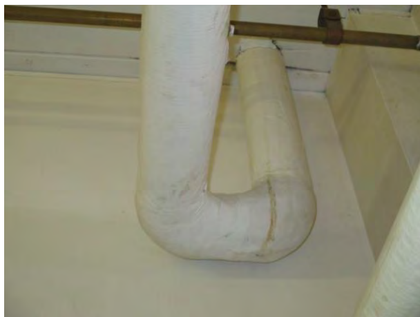
Typical pipe fitting insulation in the basement classroom (Chrysotile 40%).
