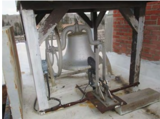
A picture showing the roof top bell and clapper system. A penetration in the roof was allowing water to enter the attic and migrate into the building, evident on both floors.
