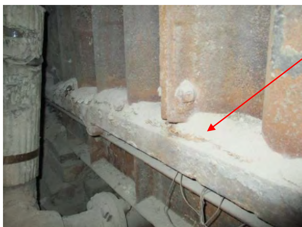
The dust and debris was collected from around the fins of the old abandoned boiler.
