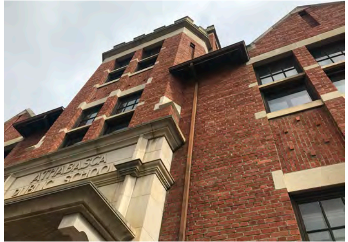
CENTRAL THREE STOREY BELL TOWER & FENESTRATION PATTERN AND WINDOWS ON CENTRAL TOWER
