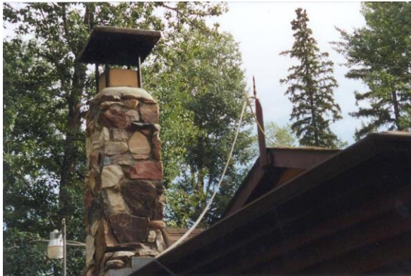
Photo 53 – Sprinklers on roof
