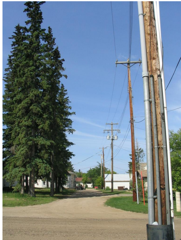
Photo 43 – Power lines overhead and low
