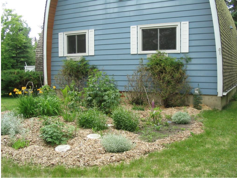
Photo 27 – Garage and home constructed of wood shake roofing and siding. East and west sides of the home are wood. Accumulation of surface fuels of wood chips in flowerbeds 5 inches thick and moss build up on the north side of the structures
