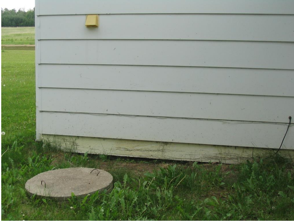
Photo 29 – Exposed insulation on base of home
