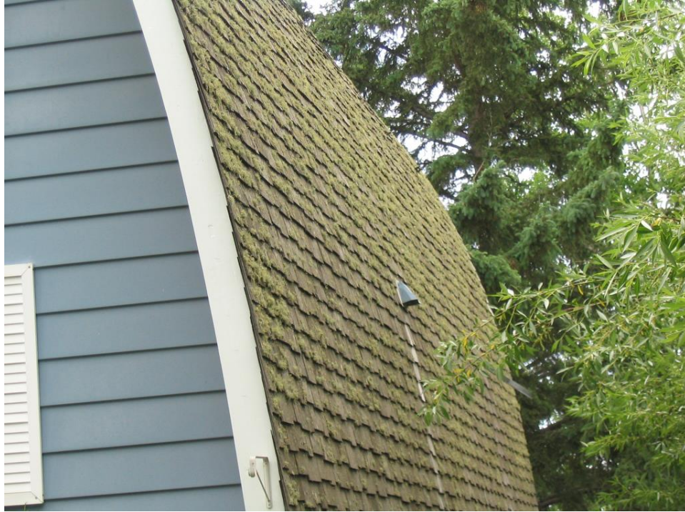
Photo 13 – Town of Athabasca: structure of unrated wood shake roofing with unrated wood shake and wood siding
