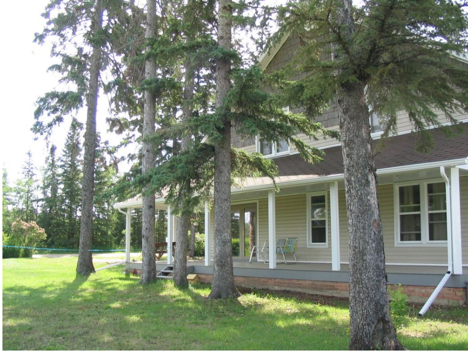
Photo 25 - Example of good defensible space of lawn or non-combustible material against structure contradicted by separated Spruce trees throughout yard that extend above roof
