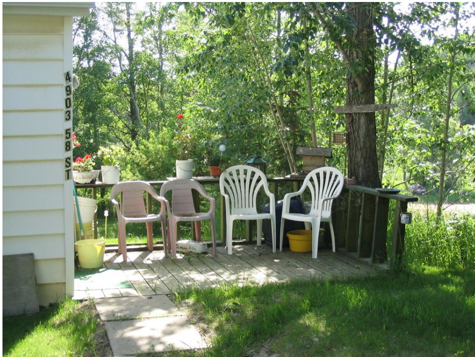
Photo 23 – Abundance of surface fuels from adjacent treed lot, wild grass and shrubs <10m from structure
