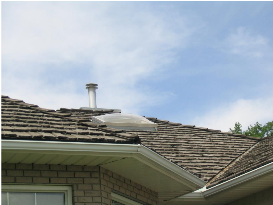
Photo 31 – Unrated wood shakes roofing
